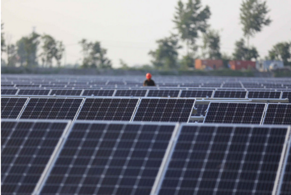
Workers install solar panels at the construction site of 40MW photovoltaic on-grid power project of China Huaneng Group in Huai an, China. | VCG/VCG via Getty Images
